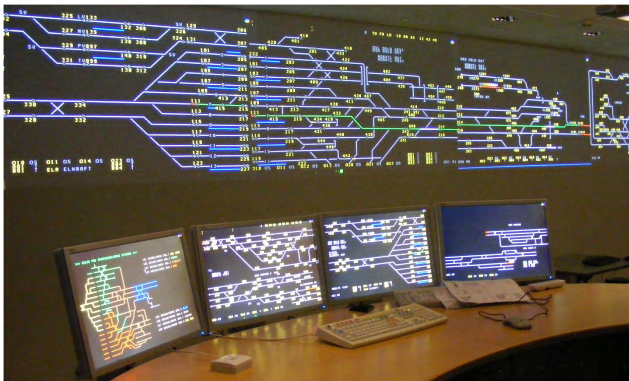
Example of previous simulator installation
